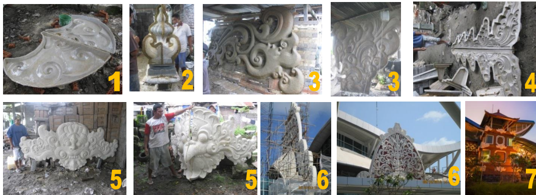
Figure 5. (1) Negative model of a mixture of silicon rubber and catalyst; (2) pour dough into mold; (3) make forms on the wall; (4) open the mold; (5) unfinished result; (6) installation on site; (7) final result
